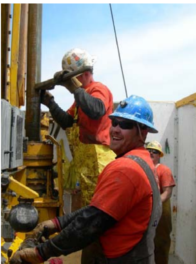
Graham Tulloch. 8 th May. Driller Shaun LaGrange with the DOSSEC team handling the drill pipe at the base of the rig.
