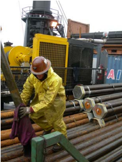
Photo 4, Graham Tulloch. DOSSEC driller Beau Marshall handling a length of drill pipe, while in the background, stacks of drill pipe are ready to be lowered down the hole.
