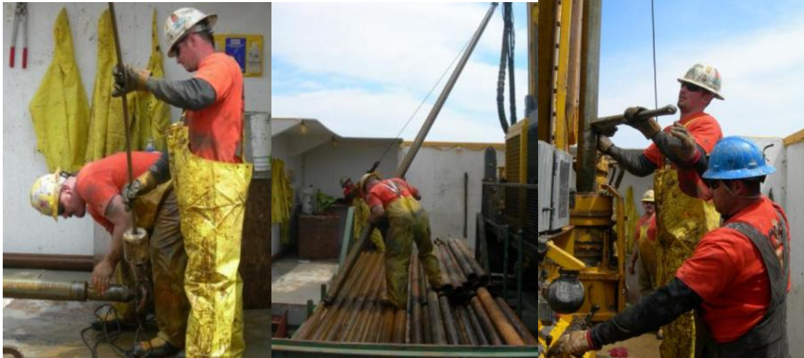
Series of photographs showing the process of running a double stand of pipe in. (G. Tulloch©ECORD/IODP).
