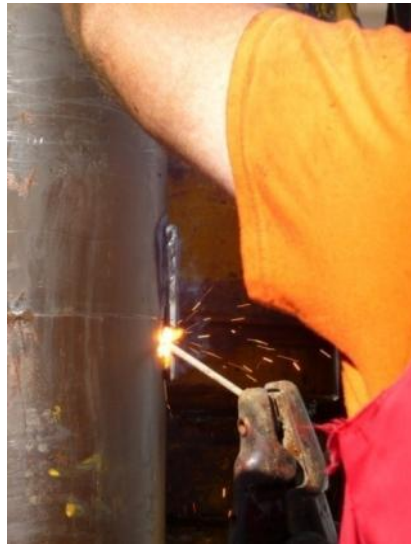
Welding tabs across the joints in slick casing to help prevent any unscrewing caused by rotation during drilling (C.Cotterill©ECORD/IODP).
