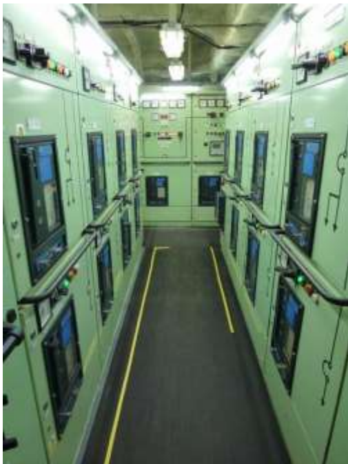
The switchboard room for the whole ship
