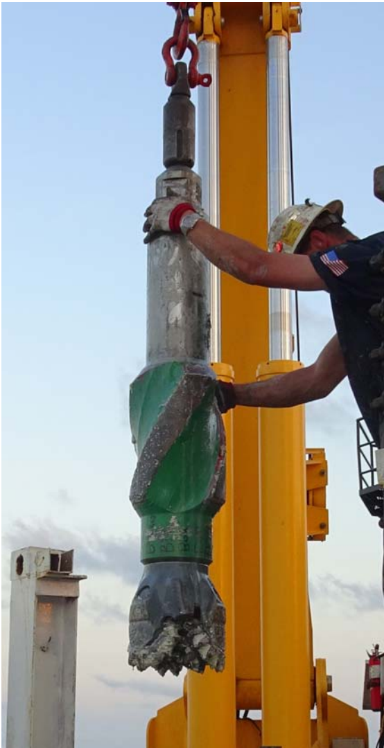
Photograph by Dave Smith © ECORD/IODP Removal of 12 ¼" Tricone drill bit, after making the hole for the conductor casing.
